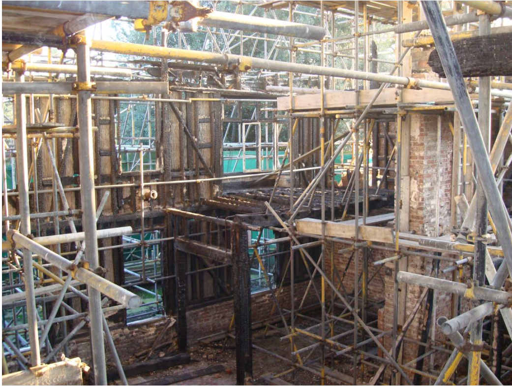
Figure 33: Interior, fire damage
