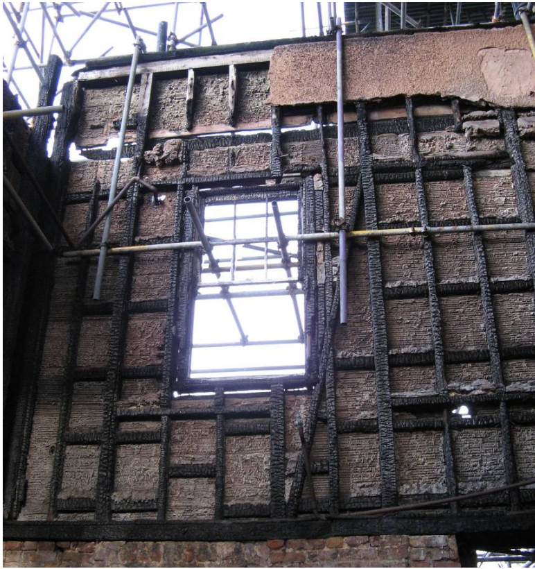
Figure 31: F4 fire damaged timber framing
